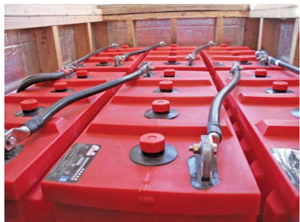
A large battery bank requires a large charging source.
