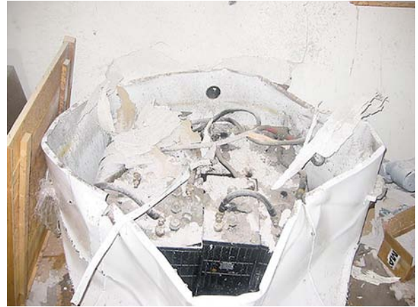
An extreme result of battery neglect.
