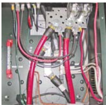
Use bus bars to parallel multiple series strings.
